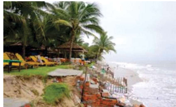
Erosion at resort on Cua Dai beach 38
